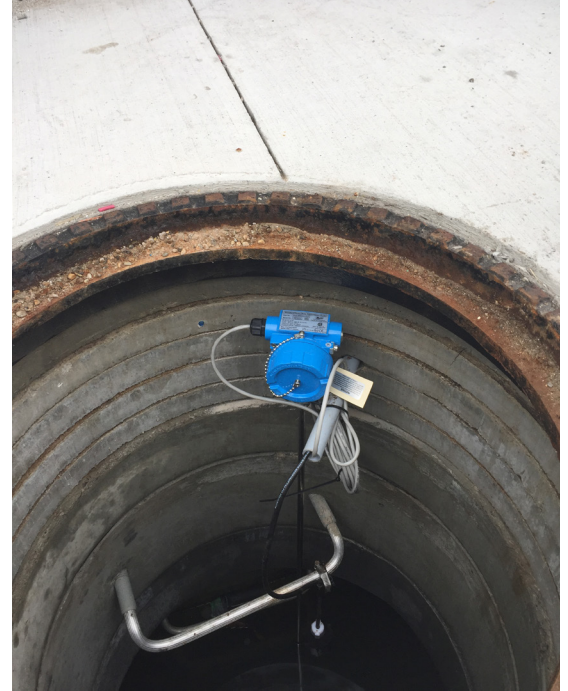
2852-OWS Oil/Water Separator Alarm Installation, Canada
