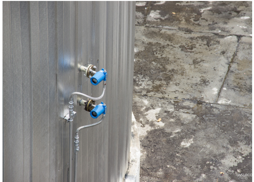
2880-OWI Oil/Water Interface Transmitter Installation, Colombia
