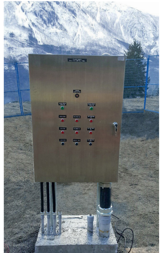
Custom control panel, British Columbia, Canada
